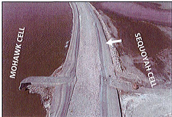
Photo 4 – showing the typical existing berm at the East Gate Berm Structure. White arrow shows approx. project location. Mohawk Cell has drawdown to 595.00 and Sequoyah Cell near empty.
