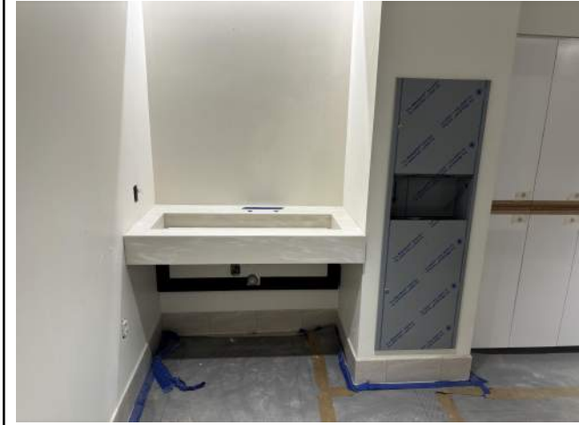
Trough sinks installed at LL1 & L1 (LL1 pictured).
