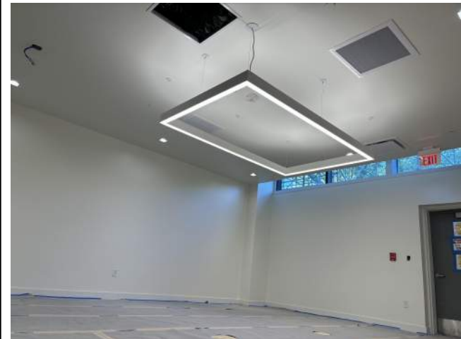
NAGPRA light installed.
