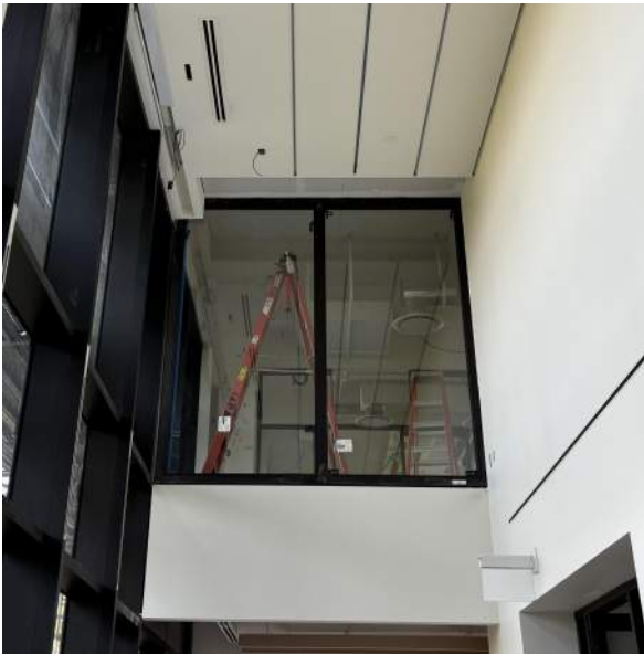
LL1 CEO Office fire rated-window in place.
