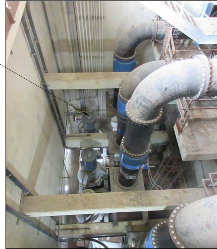
2 PHOTO – EXISTING MAIN LIFT STATION 20 SCALE: 1/8" = 1'-0"
